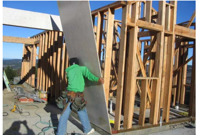
Workers apply Blazeguard (white face) sheathing using standard construction tools and practices.
