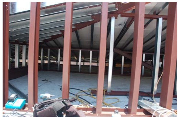
The school's new pitched roof (3 on 12 pitch) will provide stronger weather, fire protection than before.
