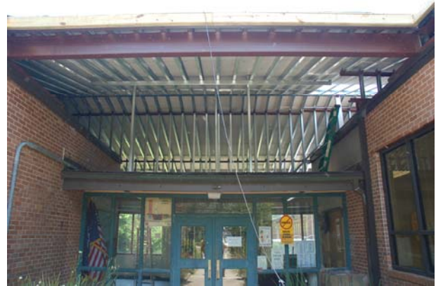
Blazeguard® (white side facing down or in) lines the interior roof of this canopy at a junior high school in Louisiana.
