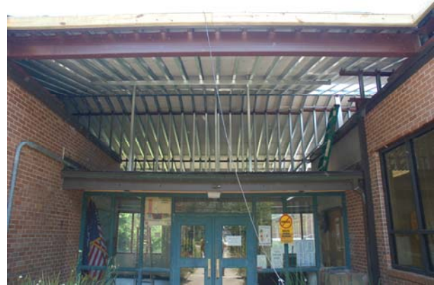
Blazeguard® (white side facing down or in) lines the interior roof of this canopy at a junior high school in Louisiana.
