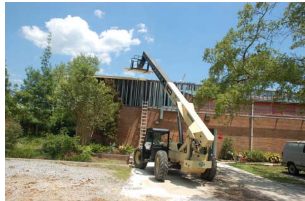
Blazeguard® Fire-Rated Sheathing is lifted to the rooftop of the school for new roof construction.
