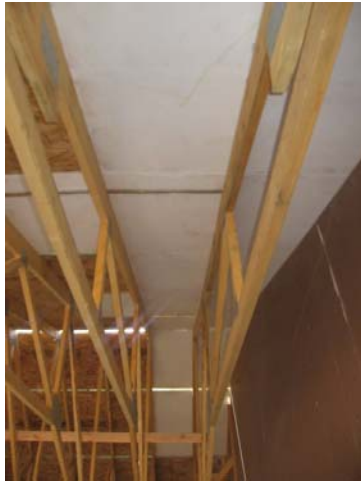
Figure 2: Blazeguard (white side facing “in” or “down” from roof) lines a party wall for a minimum of four feet.
