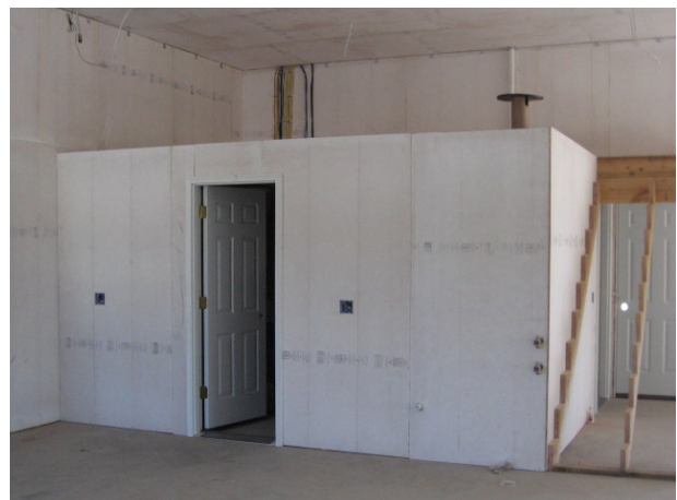
Blazeguard® secures the garage's electrical control room. Code officials can readily recognize the Blazeguard stamp.
