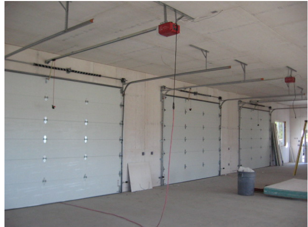
Blazeguard® (white side facing in) protects the walls and ceilings of this new shop garage
