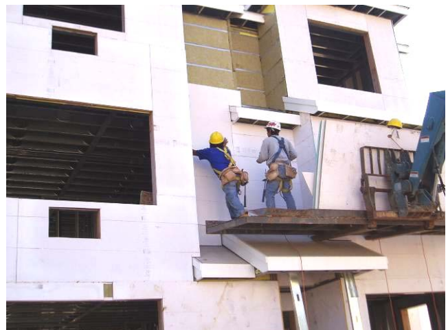
Workers apply Blazeguard (white face) sheathing using standard construction tools and practices.
