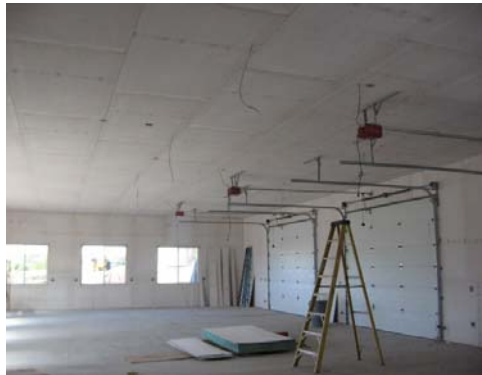
This shop garage has reveal seams.
