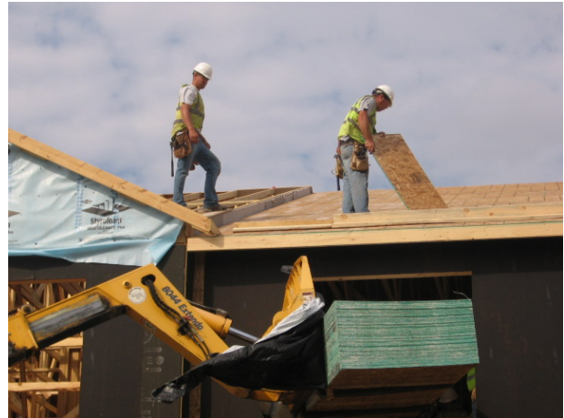
Blazeguard® Fire-Rated Sheathing being lifted onto and placed on a townhome roof deck.
